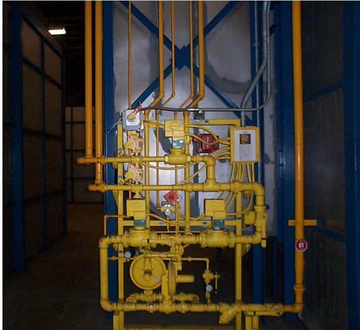
Typical Gas Train, with Flame Safety Upgrade
